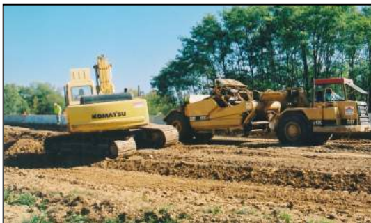
Intersection improvements are currently being made to add turning lanes and improve geometry along SR 73 through the Township.
